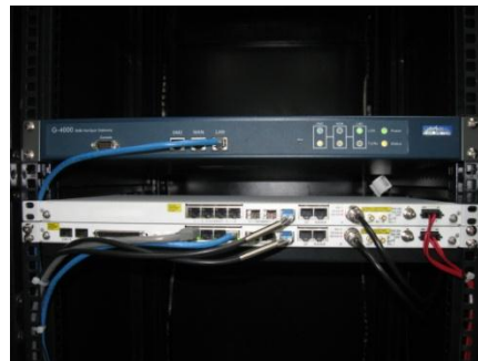
Comba equipment installed on customer site
