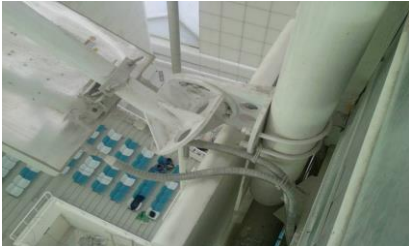
Fig 10: Venue restrictions on welding and drilling meant antenna mounts had to be customized
