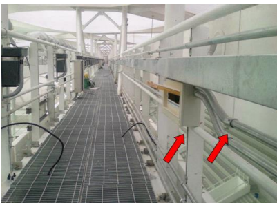
Fig 11: Prica tubing was used to protect feeders
